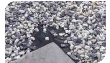
Too little aggregate
