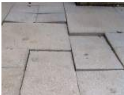
Poor bedding layer
