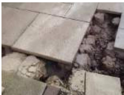
Spot bedding giving poor support
